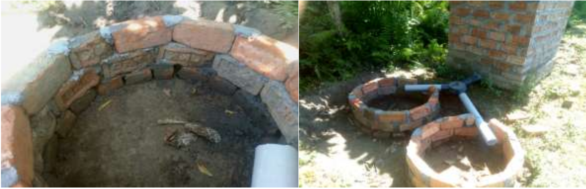
Fig- 4: Poor construction of IHHL
